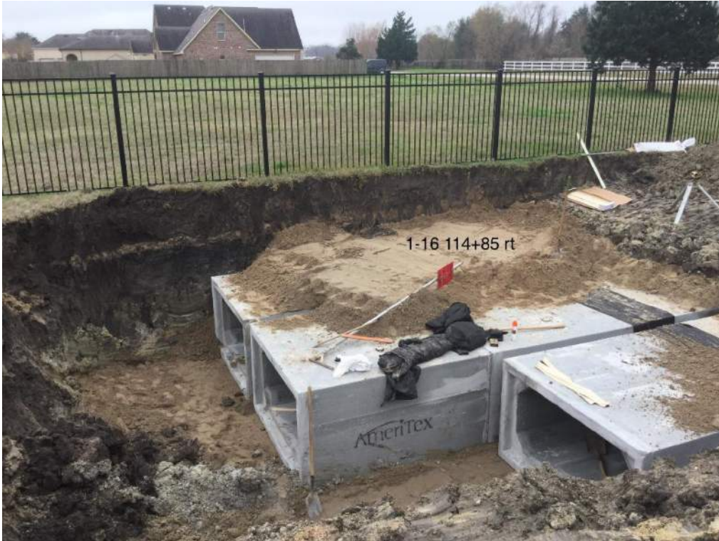
Underground detention along south ROW of Hughes Ranch Road. 01/16/2020
