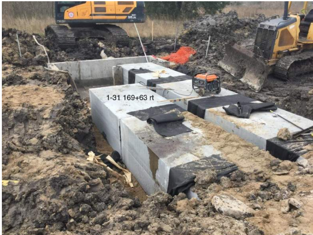
Manifold at end of underground detention. 01/31/2020
